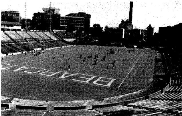
Voids beneath the stadium, resulting from subsidence of the original (1920) earth form were filled with Ultra-Lite 220. To ensure continued spectator safety and add years to the life expectancy of the structure. — Cincinnati, Ohio
